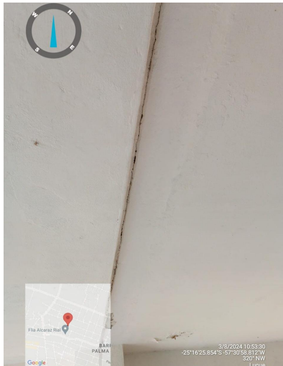
Annex 8: Defects detected in the classroom.
