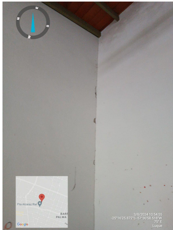
Annex 6: Deterioration noted in the classroom.
