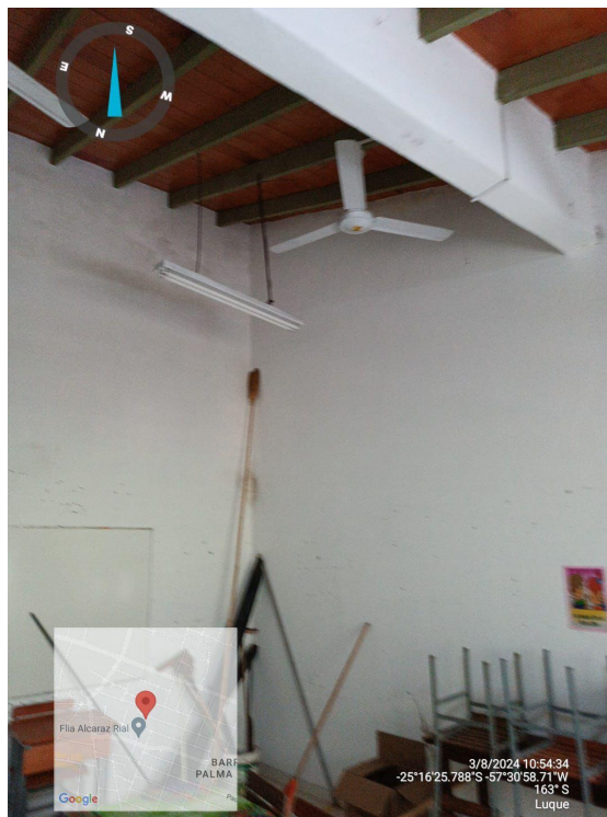
Annex 9: Alterations observed in the classroom.
